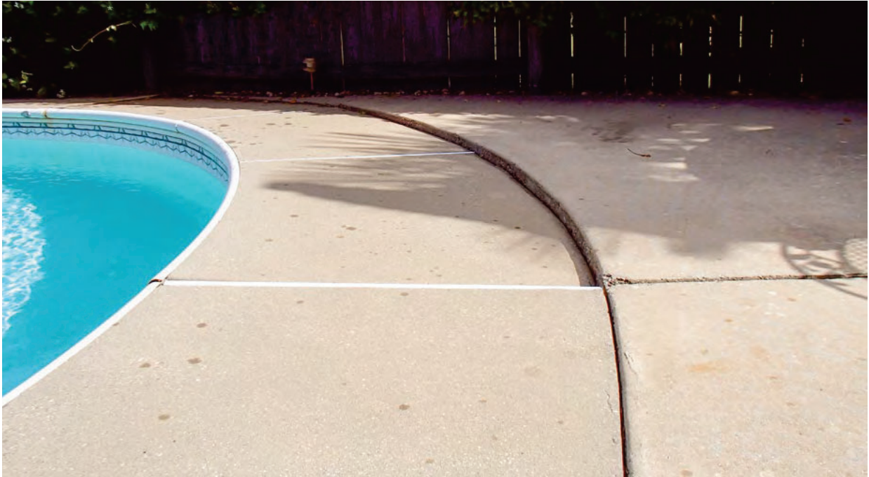
Figure 5.5 Pool deck slab settlement
